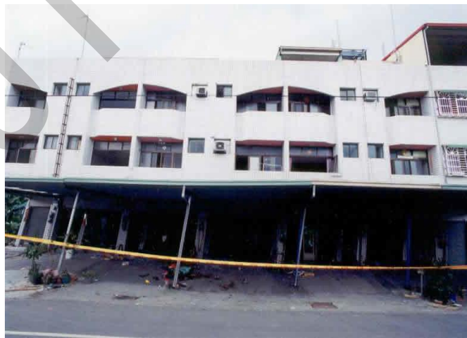
Figure 1: General Mode of Failure in OGS Buildings
